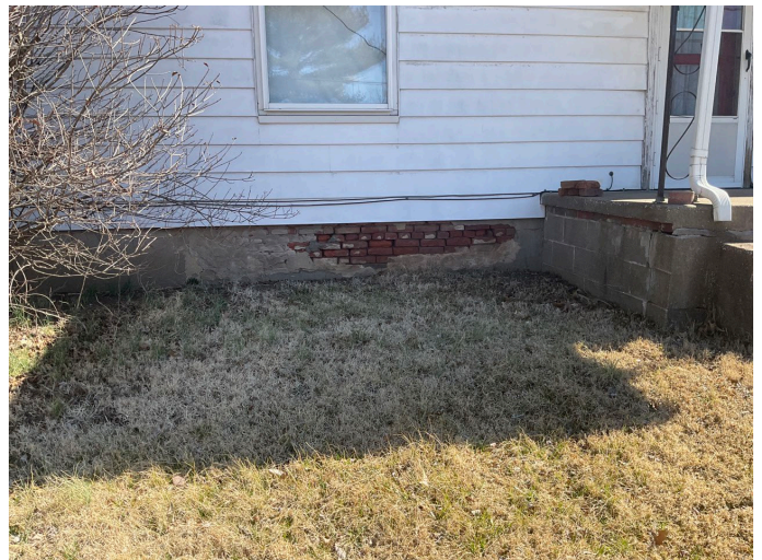
Deteriorated masonry foundation at 414 N. Market Street.
