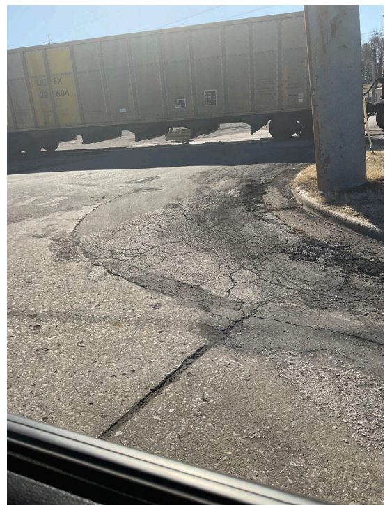
Deteriorated street pavement on S. Vine Street at rail road intersection looking south.
