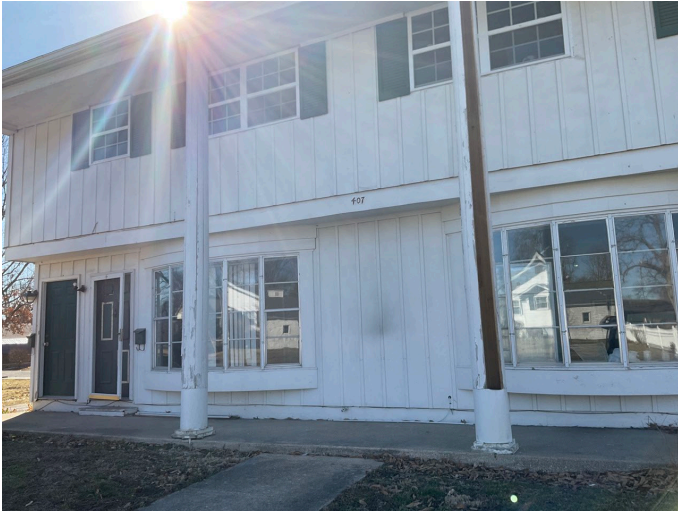
Deteriorated siding, columns, and windows at 407 S. Oak Street.
