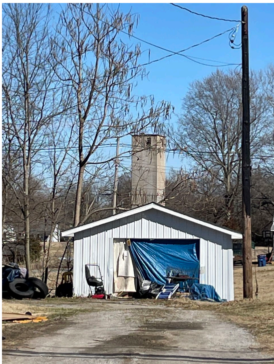
Deteriorated detached garage at 218 N. Market Street has a missing roll-up replaced by tarp. April 2022
