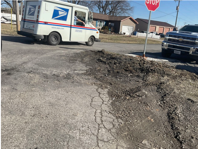
Intersection of N. Vine Street and E. Hood Street: Deteriorated pavement, lack of curbs and gutter, and no sidewalks.
