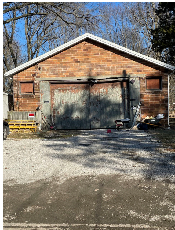
Deteriorated windows and door on detached garage at 412 S. Wilson Street.
