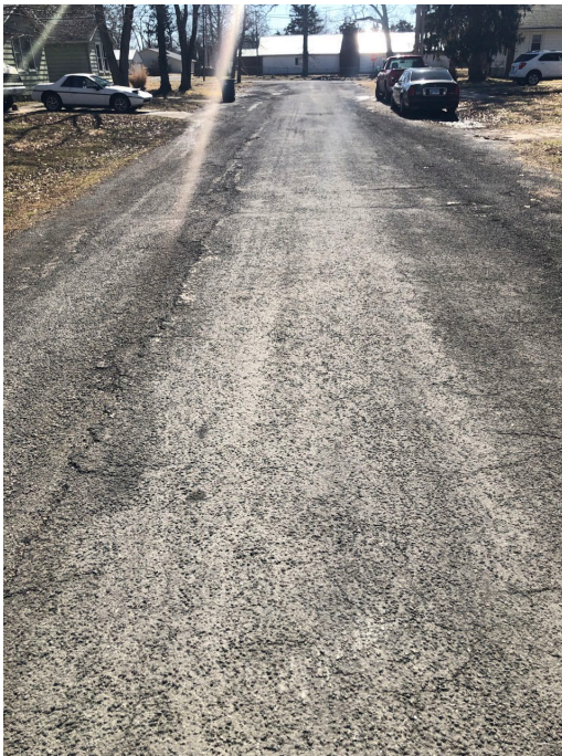
S. Walnut Street between W. Grigg Street and W. Belmont Street: Deteriorated pavement, lack of curbs and gutters, and no sidewalks.
