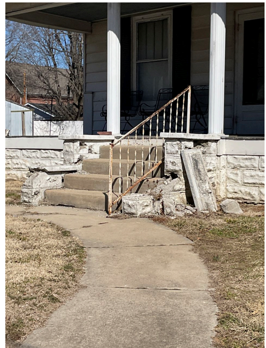
Deteriorated porch stairs and railing at 308 N. Market Street.
