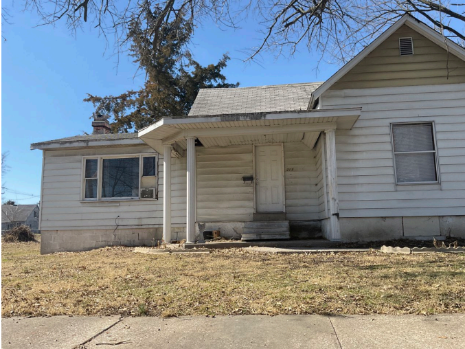
Deteriorated soffit, fascia, windows, and siding at 313 N. Washington Street.
