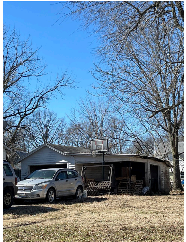
Deteriorated roofing, soffit, fascia, and siding on detached garage at 614 N. Vine Street.
