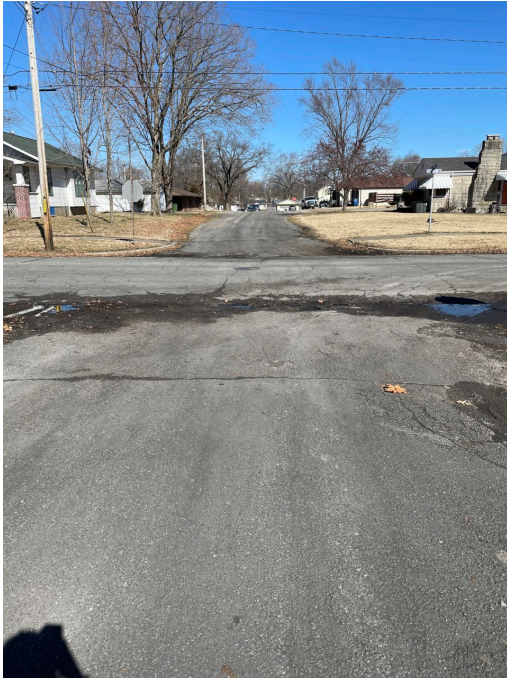
Intersection of S. Gordon Street and W. 3 rd Street: Deteriorated pavement, curbs and gutters.
