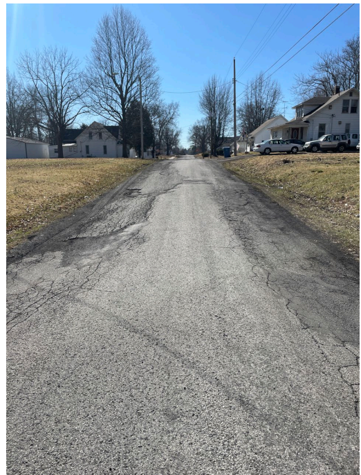
E. Sproul Street between N Vine Street and N. Washington Street: Deteriorated pavement, lack of curbs and gutters, and no sidewalks.
