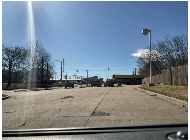
Deteriorated parking area and obsolete fuel dispensing equipment at 201 E. Broadway Street; a vacant retail storefront which was previously a gas station.
