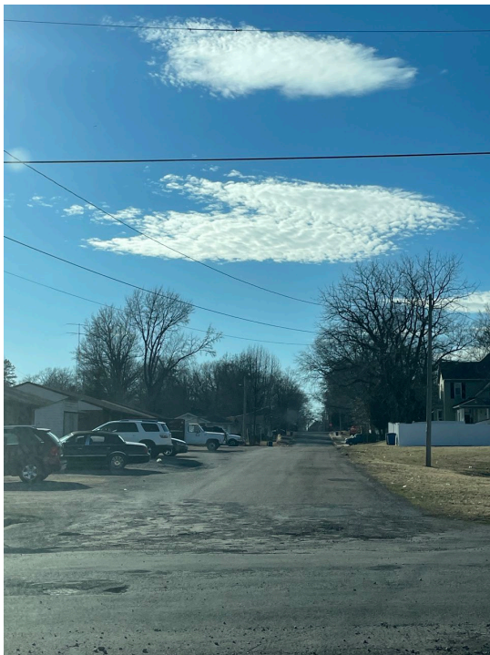
3 rd Street between Market Street and Vine Street: Deteriorated pavement, lack of curbs and gutter, and no sidewalks. April 2022
