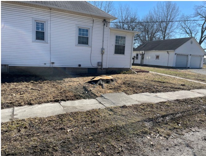
S. Gordon Street between W. 3 rd Street and W. Belmont Street: Deteriorated sidewalks and lack of curbs and gutters.
