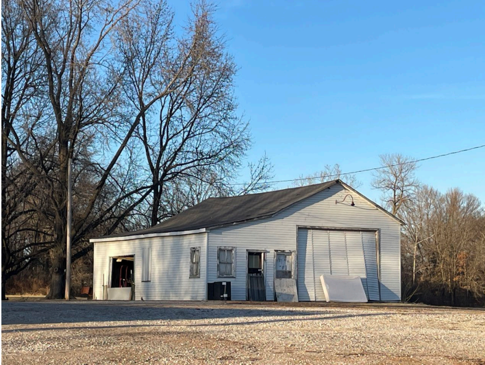
Deteriorated windows, doors, siding, and fascia on accessory structure at 700 S. St. Louis Street.
