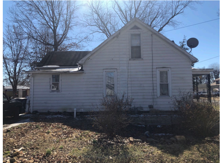
Deteriorated roofing, soffit, fascia, gutters, windows, and siding at 500 S. Walnut Street.
