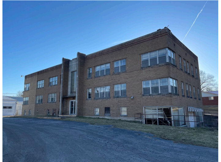
Deteriorated windows and masonry at 615 S. St. Louis Street.
