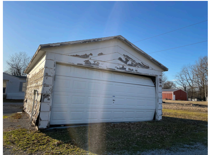
Dilapidated detached garage at 903 St. Louis Street shows signs of buckling exterior walls, deteriorated siding, fascia, soffit, and door.
