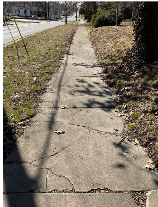
Deteriorated sidewalks on S. St. Louis Road between W. Belmont Street and W. 3 rd Street.
