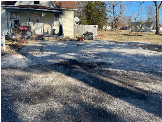
Deteriorated off-street parking area at 412 S. Wilson Street.
