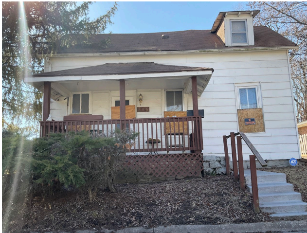
Deteriorated roofing, fascia, porch and foundation at vacant residence at 109 S. Washington Street.
