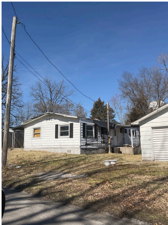
Dilapidated structure at 209 E. Mound Street shows apparent fire damage. April 2022
