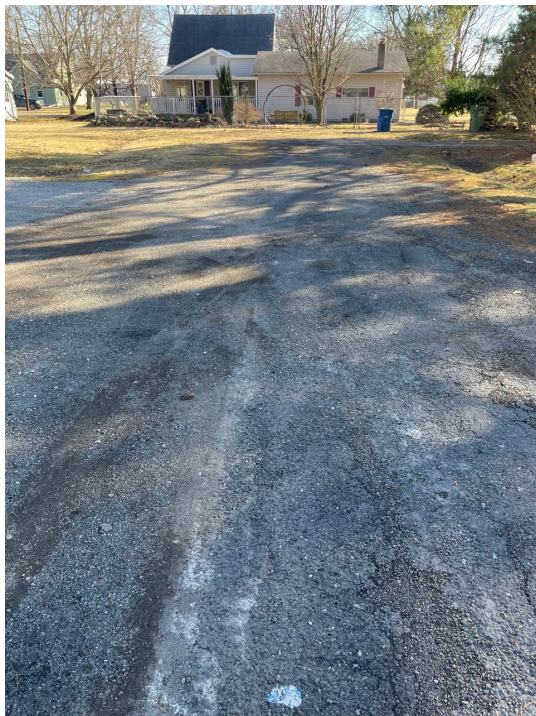
S. Wilson Street: Deteriorated pavement, lack of curbs and gutters, no sidewalks, and dead-end street lacking modern cul-de-sac roadway design.
