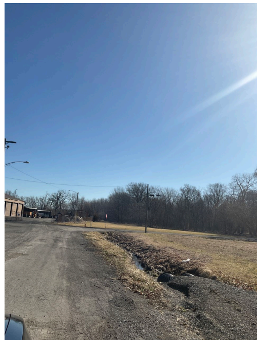
E. Hood Street between N. Vine Street and N. Washington Street: Deteriorated pavement, lack of curbs and gutter, no sidewalks, and deteriorated stormwater drainage facilities.
