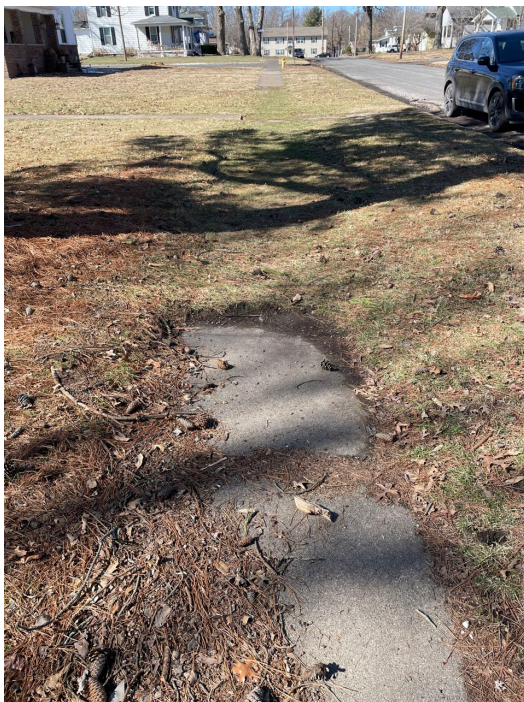
Deteriorated Sidewalks on W. 3 rd Street near intersection of Belmont Trail Ct. April 2022
