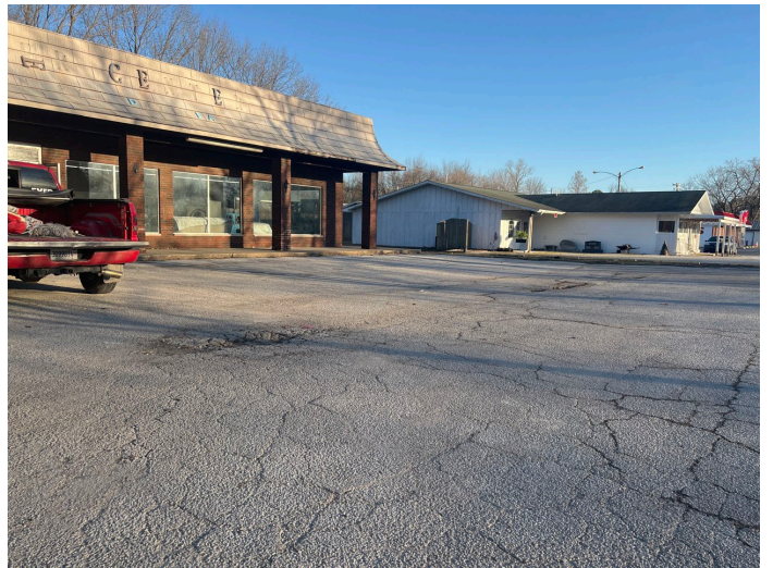
Deteriorated parking area at 912 S. St. Louis Street.
