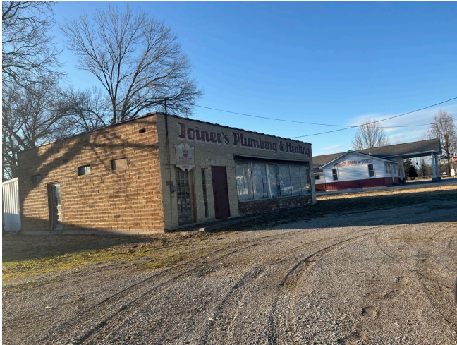
Deteriorated driveway at vacant retail storefront on west side S. St. Louis Street between Delinda Avenue and Janet Avenue, adjacent to 903 S. St. Louis Street.
