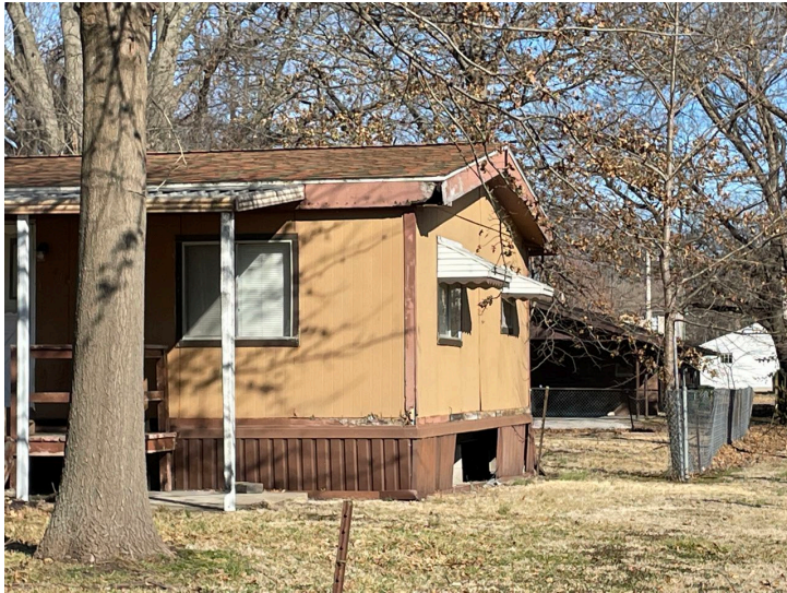
Deteriorated porch decking, siding, and skirting on mobile home structure at 410 S. Grand Avenue.
