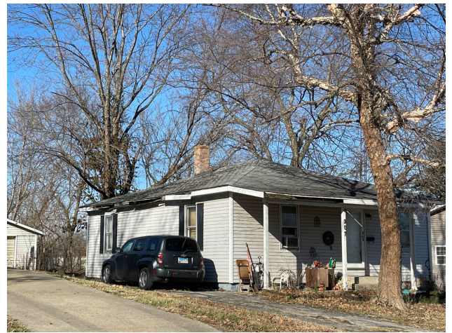
Deteriorated roofing, soffit, and fascia at 207 E. 2 nd Street.
