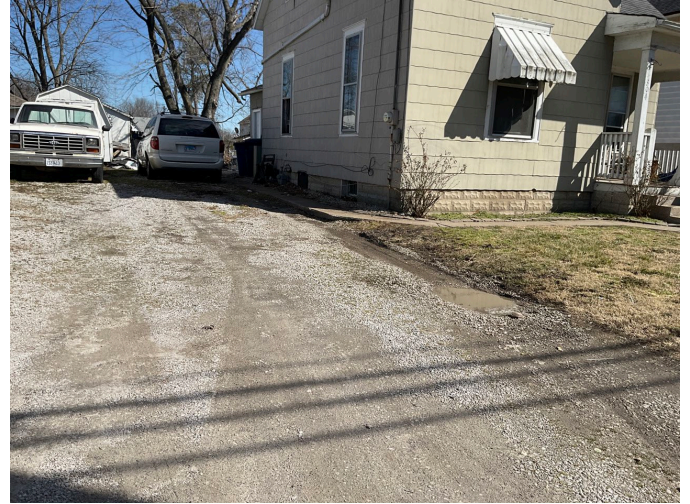
Deteriorated driveway at 304 N. Market Street.
