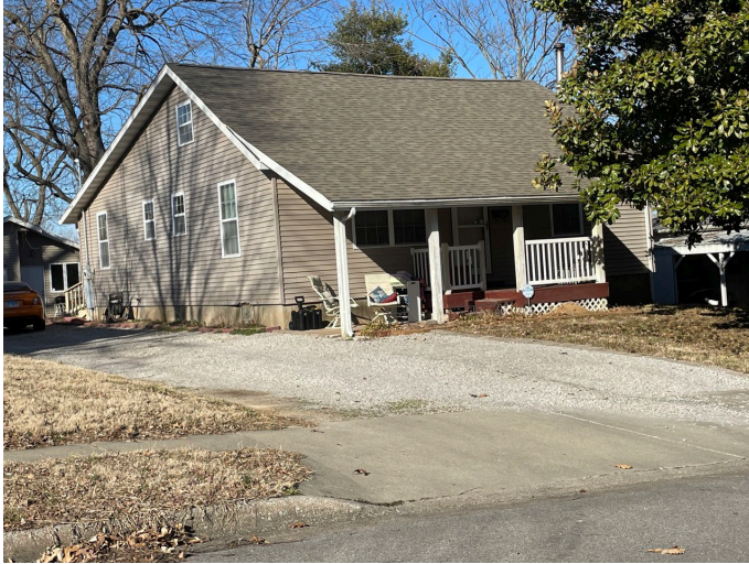
Deteriorated driveway at 209 E. 2nd Street.
