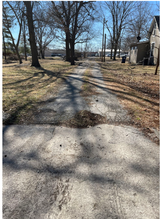
Belmont Trail Ct. looking south from W. 3 rd Street: Deteriorated street right-of-way exhibiting deteriorated pavement, lack of curbs and gutters, and no sidewalks.
