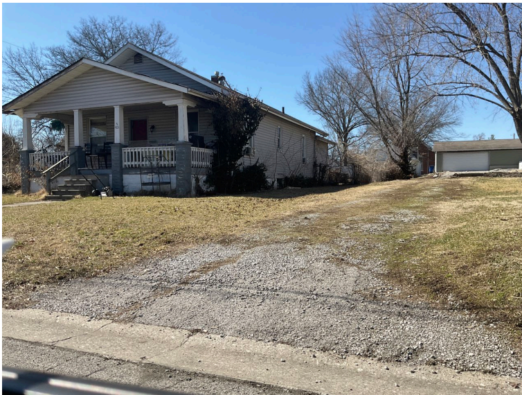
Deteriorated driveway at 401 N. Washington Street.
