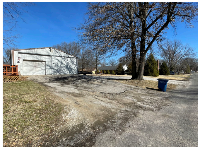
Deteriorated driveway at 600 N. Vine Street.
