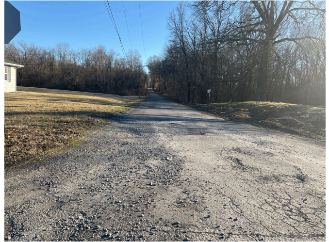
Intersection of 4 th Street and Deer Creek Lane: Deteriorated pavement, lack of curbs and gutter, and no sidewalks.
