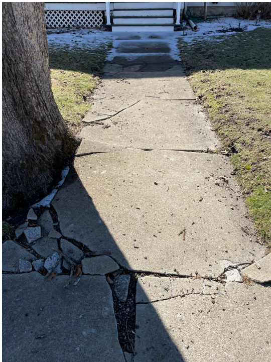
Deteriorated sidewalk at 400 W. 3rd Street April 2022
