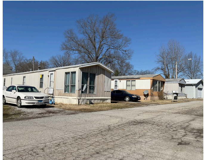
Deteriorated siding and skirting on mobile home structures at 1-4 Belmont Trail Ct, a parcel also exhibiting excessive land coverage.
