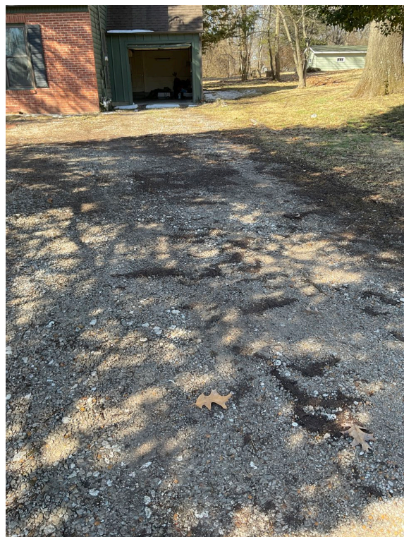
Deteriorated driveway at 517 S. St. Louis Street.
