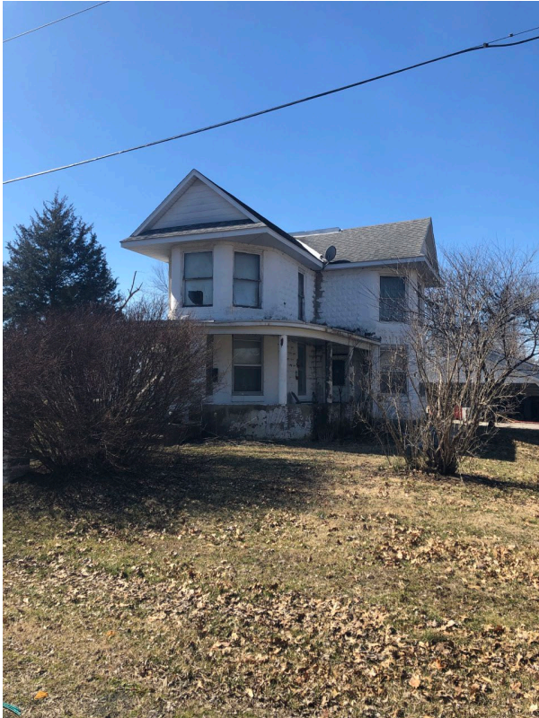
Deteriorated porch, windows, and masonry at 501 S. Walnut Street. April 2022
